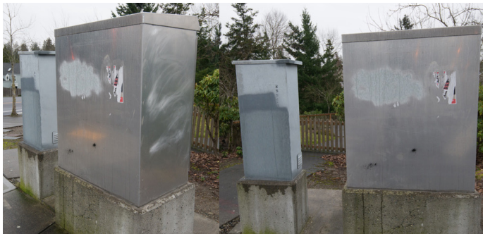
This is the actual box to be wrapped with CATS artwork. The location is 312th and 23rd.
